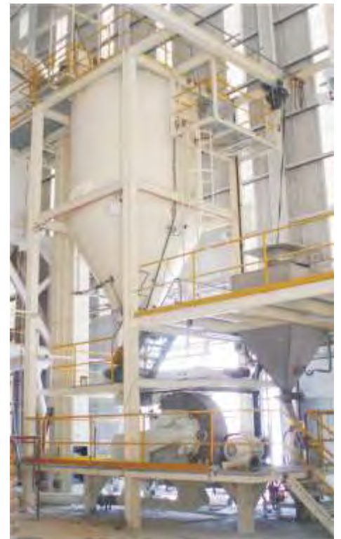
SIERRA 63 in a coating installation
