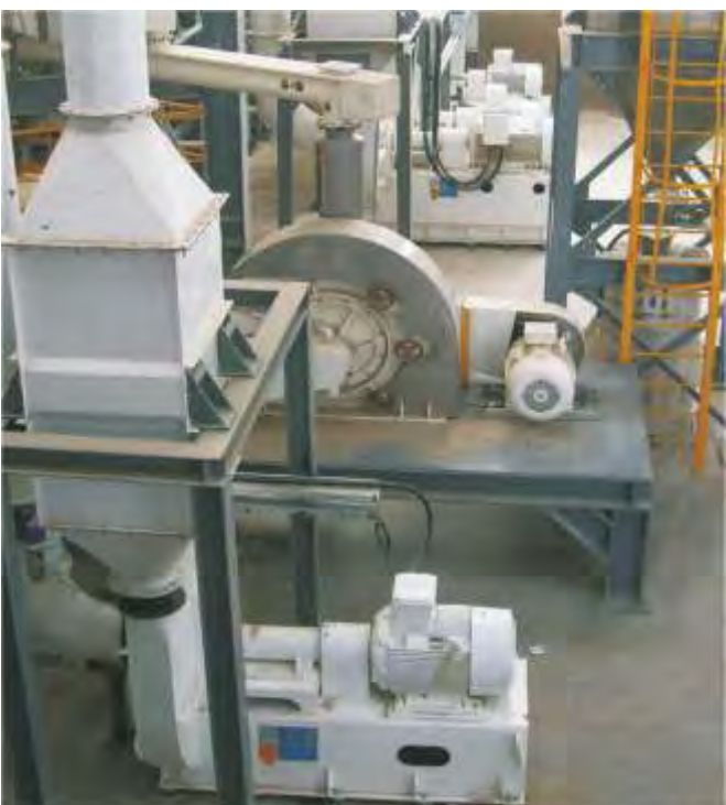
SIERRA 63 in a coating installation
